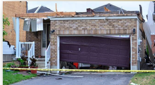
Damage from the Angus Ontario Tornado 2014
