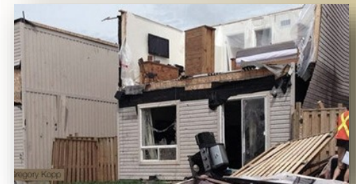
Damage from the Angus Ontario Tornado 2014
